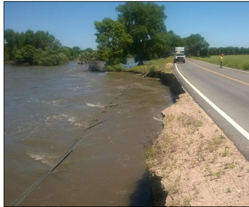
Figure 3-4: Colorado State Highway 144, near Orchard, Colorado, following the September 2015 flooding (CDOT 2015)
